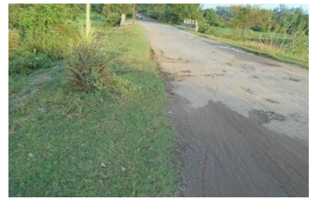
Cleaned road at CR 45 near Bridge
